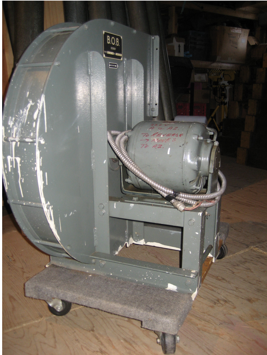
B.O.B. Blower and motor
